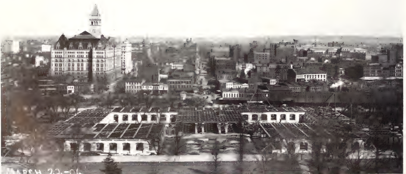
Foundation of the new National Museum, probably taken from the tower of the Smithsonian Castle. The low area in the center is the site of the Baird Auditorium. March 22, 1906.
